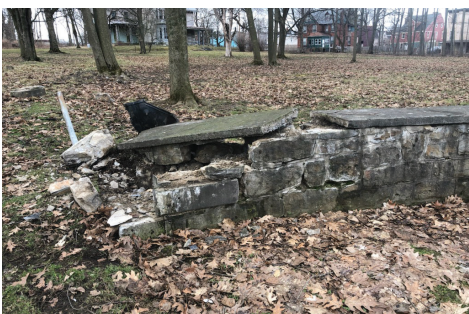
WALL DAMAGE IN FRONT OF #3 RUTGER PARK
